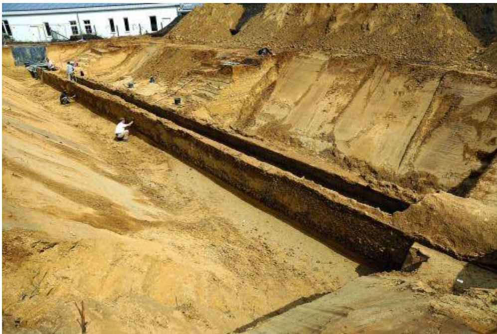
Figure 1: The well-preserved section of the Roman water pipeline near Hürth-Hermülheim during excavation. (A. Thieme/ArchaeoNet GbR)
