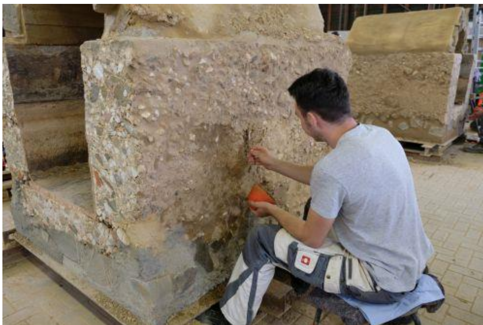
Figure 6: Trainee from the Cologne Chamber of Crafts during the restoration of a segment of the water pipeline. (Th. Sieverding)
