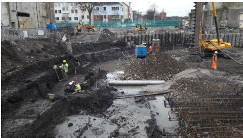
Figure 3: Excavation of the basement took place in stages in tandem with construction. The size of individual units was restricted because of sub-surface tidal pressure and access requirements
