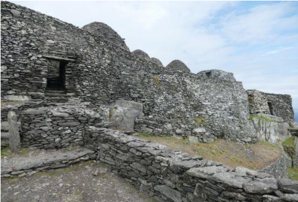
Figure 14: Monastery retaining wall in danger of collapse (Image credit: OPW)
