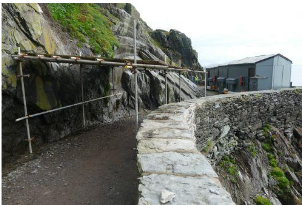
Figure 18: Temporary crash deck installed in the location of rock falls (Image credit: OPW)
