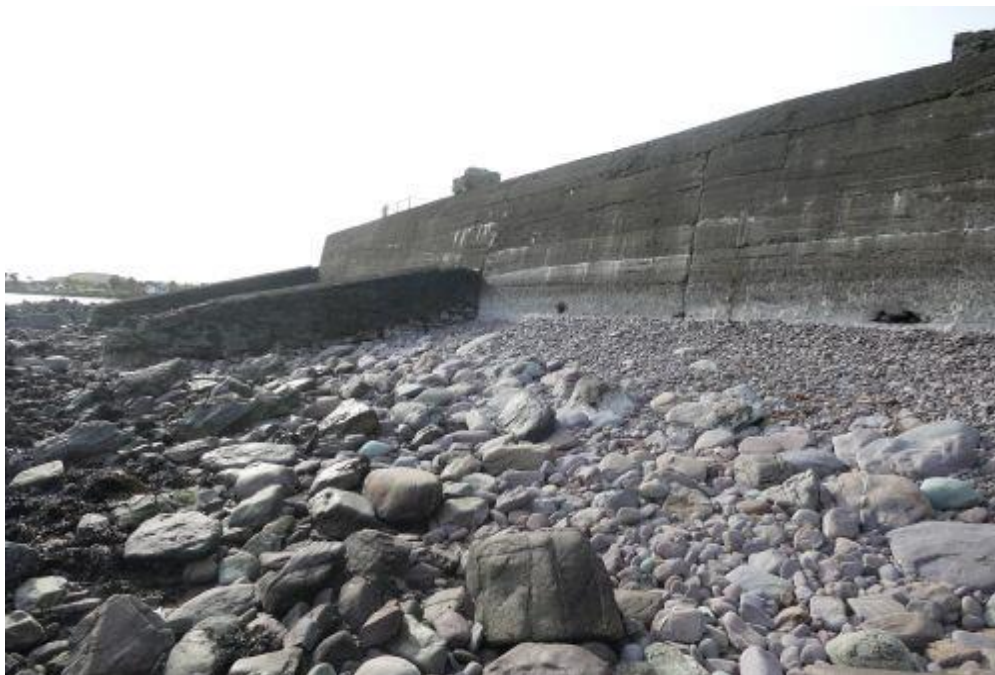
Figure 26: Erosion to existing concrete sea wall (Image credit: OPW)
