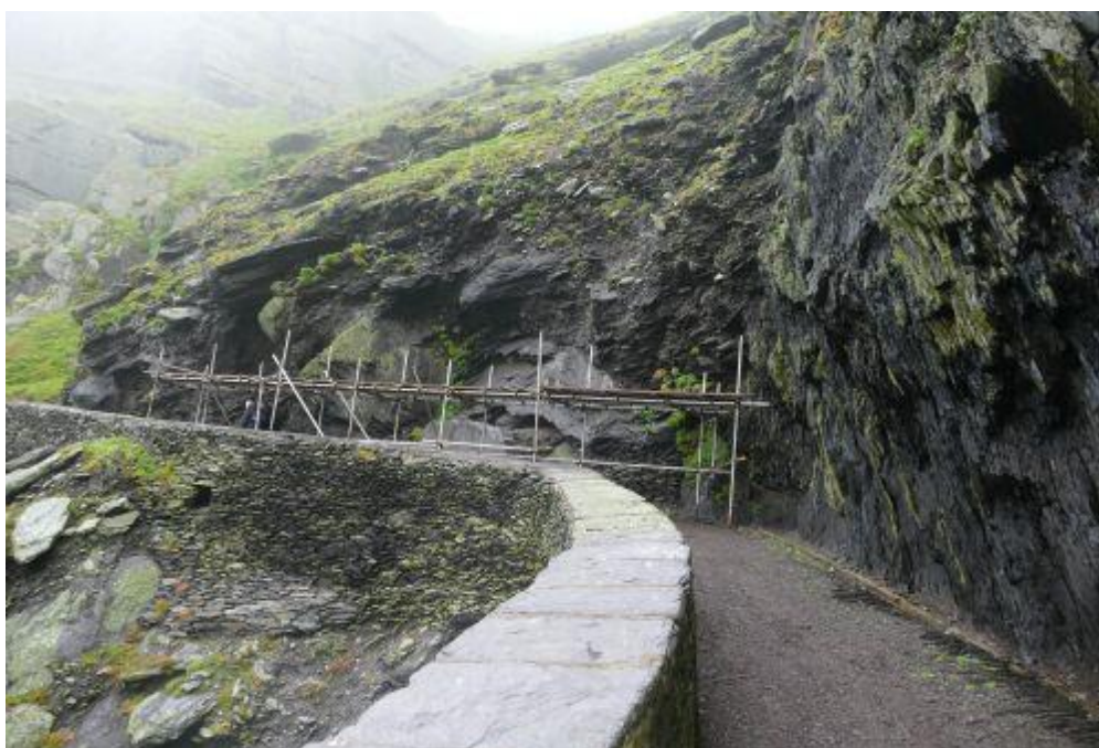
Figure 19: Temporary crash deck installed in a critical location on the Lighthouse Road (Image credit: OPW)
