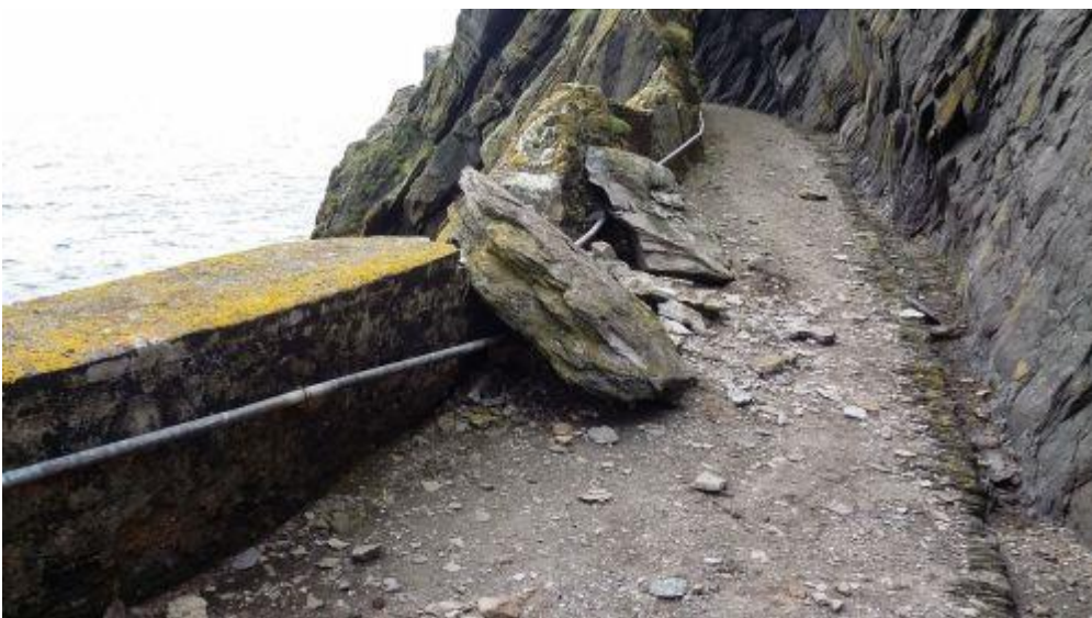
Figure 15: Rock fall in 2017 (Image credit: OPW)
