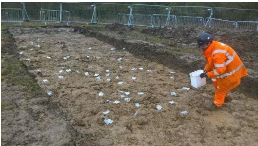
Figure 1: A trial trench in Dews Farm, Hillingdon: HS2 Phase One. Image credit: HS2 Ltd
